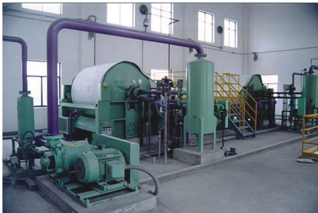
Drum Filter Vacuum System
