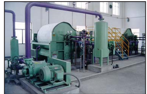
Drum Filter Vacuum System
